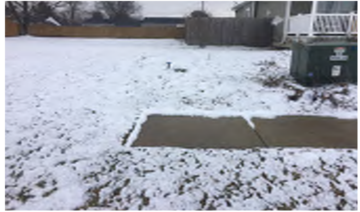
Figure 6.1 - A relatively new and high quality sidewalk ends abruptly.
